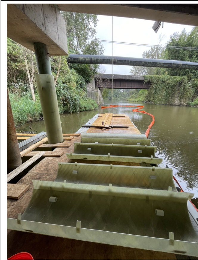
CarboShield pile encasement shells ready on the staging area underneath the INDOT U.S. 20 bridge being repaired.
