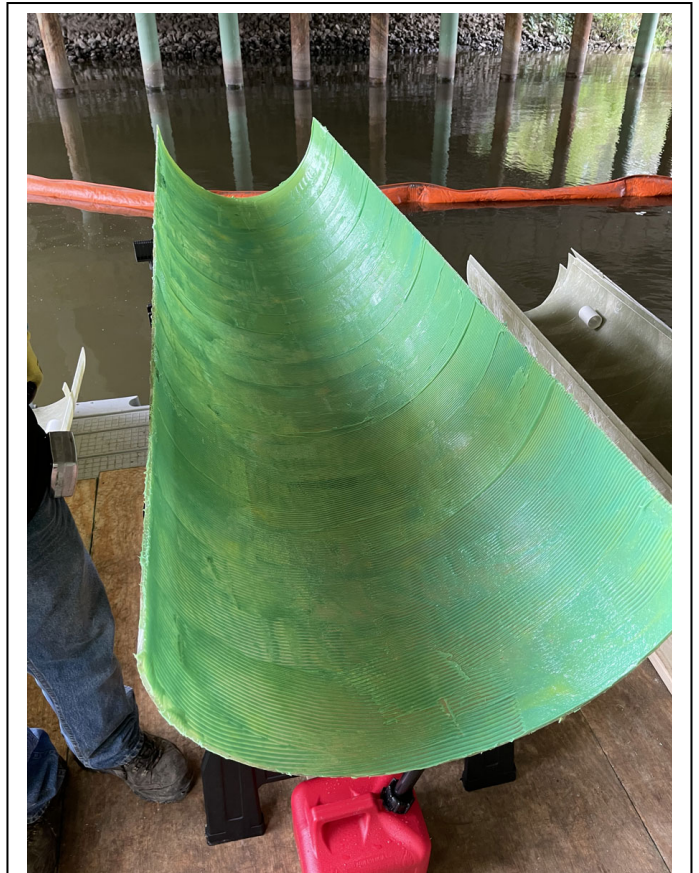
Epoxy is applied to the inner face of the outer CarboShield shell to bond the shells for full pile encasement.
